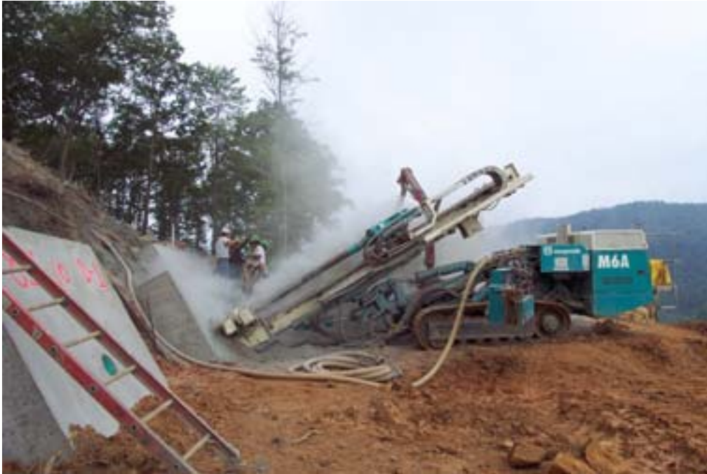
The contractor is drilling for the ground anchors. Note the anchor block set prior to drilling.
