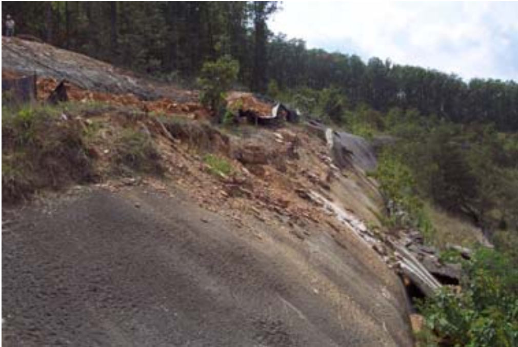
This close-up shows the damage to the existing soil nail wall caused by the slide.
